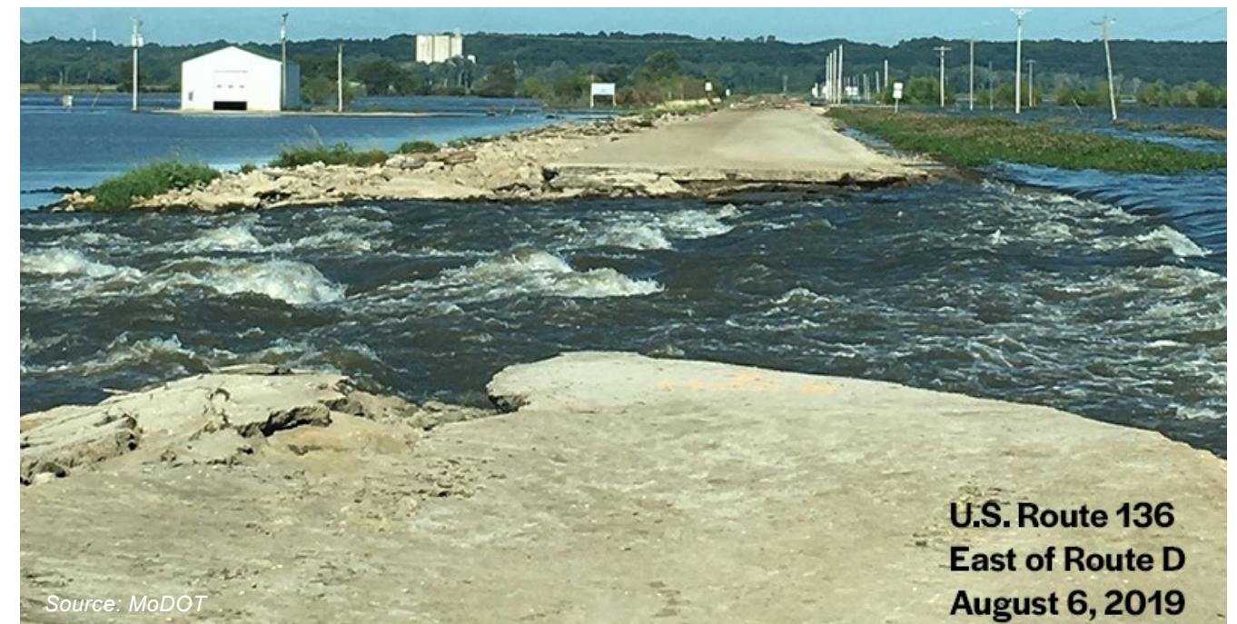
Figure 1 – 2019 Flooding Washes Out a Section of U.S. Route 136
